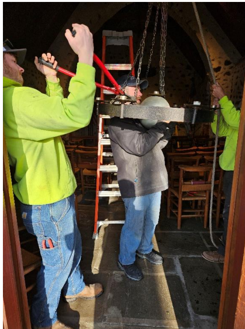
Photo 1: Three technicians bringing down alter chandelier. One holding the fixture, one cutting chain assembly, and one holding tension on offset weighted pulley system.
